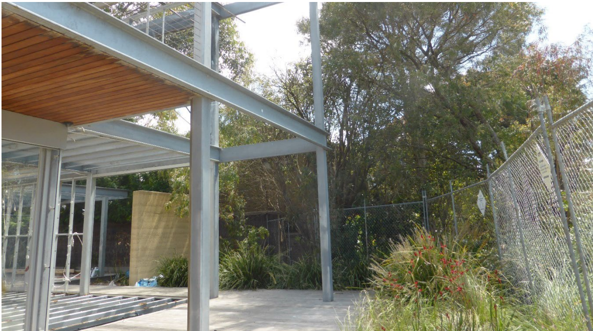
Figure 2 The batch HDG structural steel members (verandah posts and edge members) have good access and would be expected to provide structural support with regular maintenance of the galvanized coating for 50 years in moderate locations. Regular maintenance, plus repairs to the galvanized coating should be expected to be carried out during the life of the building in severe environments.
