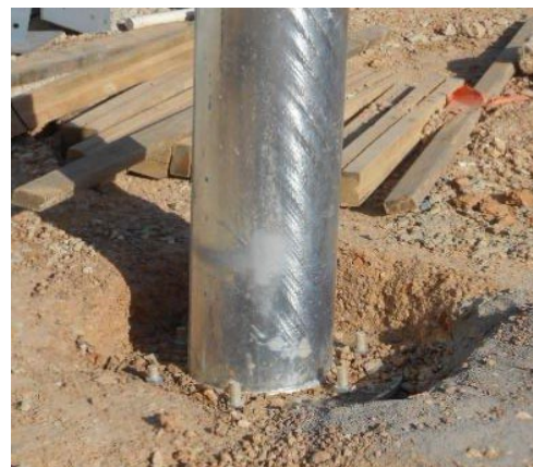
Figure 9 This large post bolted to a concrete pad will finish below the ground level and will be at risk of collar corrosion reducing the durability of the structure unless additional protection is added.
