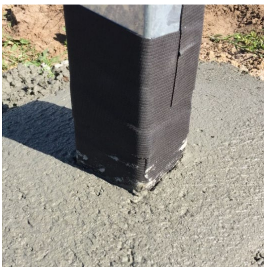
Figure 14 Denso Ultraseal tape wrapped around the base of a newly embedded post.
