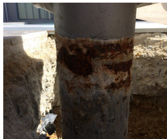
Figure 15 A galvanized post without additional protection at the steel and concrete interface showing accelerated corrosion which has reduced the overall durability of the structure. The galvanized coating above the ground remains in excellent condition.
