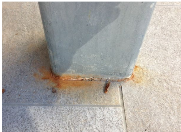
Figure 8 A verandah post embedded into a tiled floor in a wet area. Water has seeped into the gap between the tile and the steel through capillary action, leading to accelerated corrosion and early failure. This is a design defect where separation of the water from the steel was not considered.
