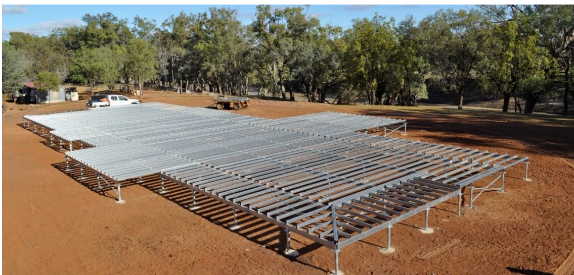
Figure 4 Batch HDG structural steel posts in combination with a continuous HDG sub-floor located in a Low (C2) environment (more than 10km from breaking surf).
