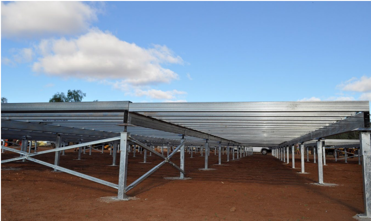
Figure 16 A pre-galvanized steel subfloor (with inbuilt ant caps) in a Low (C2) environment with the batch HDG posts bolted down onto elevated concrete pads.
