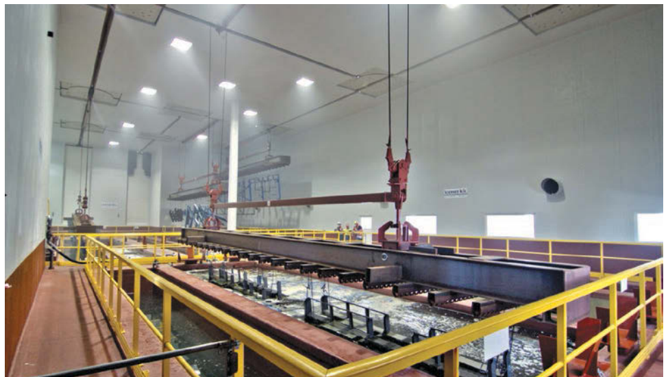
Enclosed pre-treatment area with extraction fans to capture all emissions.
