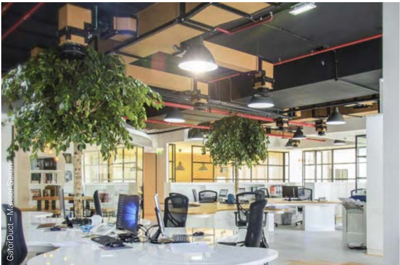
Figure 104: Example of cardboard ductwork, Gatorduct, used in an office environment
