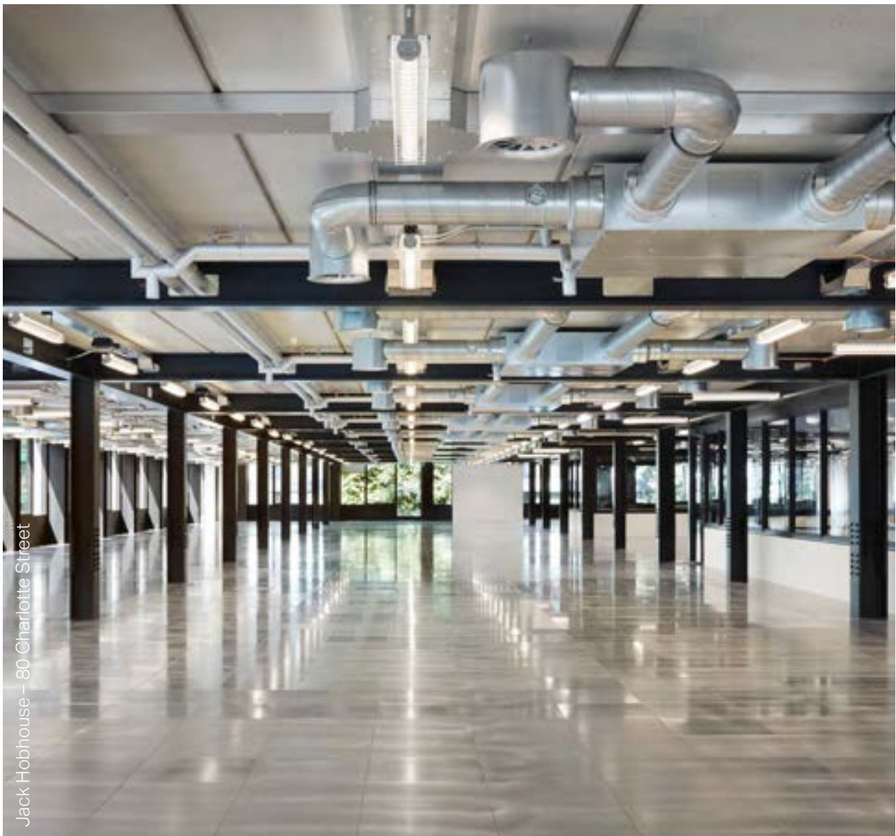
Figure 106: Example of exposed services in 80 Charlotte Street, London
