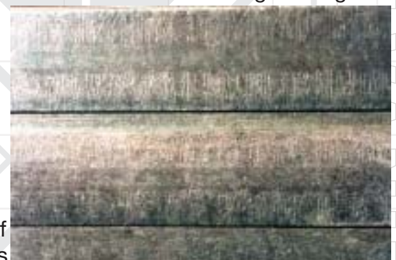
These lateral striations are a result of surface stresses in the steel section cause by the rolling process reacting at a higher rate with the molten zinc than the surrounding steel.
