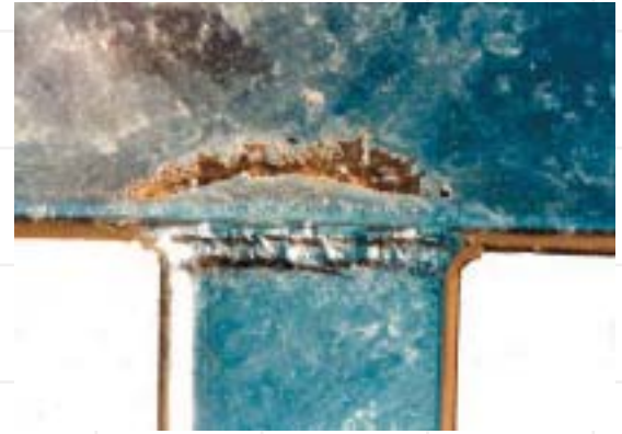
This miss in the galvanized coating is caused by surface contamination by residual oxides not removed in the pickling process.
