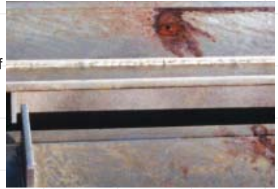
Flux staining has occurred on unsealed vent holes in overlaps on this fabrication. The stains are caused by iron salts, that have penetrated the overlap during pre-treatment, re-hydrating with atmospheric moisture.
