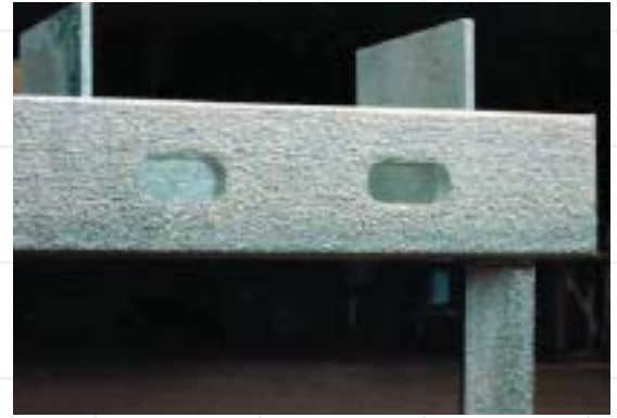
The textured surface on this steel angle results from the rough as-rolled surface of the base steel, usually cause by excessive mill-scale on the steel section in the hot rolling process.
