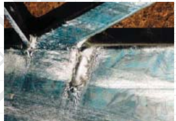
Zinc run caused by zinc freezing while draining from flat RHS surface. Durability is enhanced but thick runs may interfere with connecting surfaces
