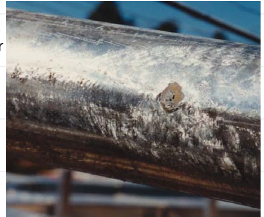
Where jigs are used to support large items in the galvanizing processes, touch marks will occur where the galvanized coating adheres to the jig at the point of contact.
