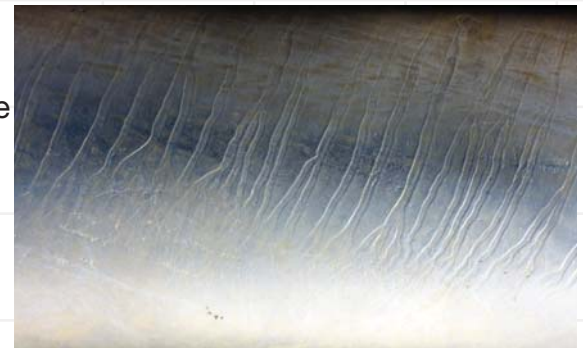
Fishbone striations on large diameter pipes arise from surface stresses in the steel causing different zinc-steel reaction rates on the pipe surface.
