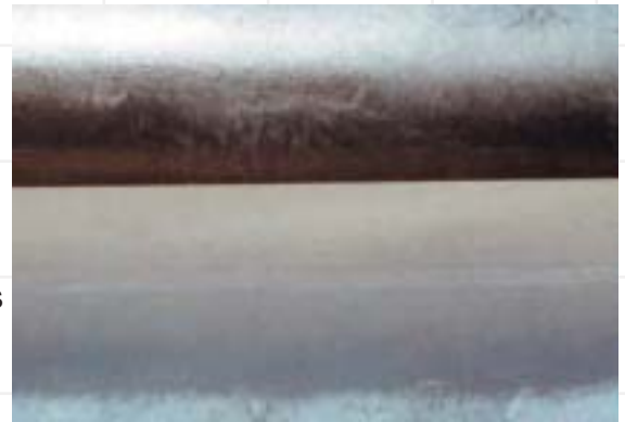
The gray coating on these pipes is a result of high silicon content of the steel, making it more reactive and converting all the coating to zinc-iron alloy. These gray coatings are typically thicker than shiny galvanized coatings on similar sections.
