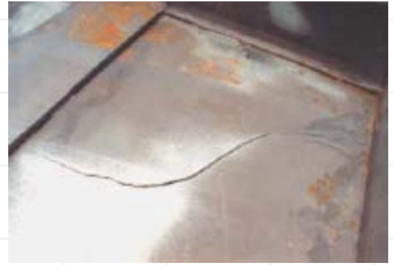
The fracture of Bisalloy wear plate is a result of Hydrogen embrittlement arising from the pickling process. High strength (over 800 MPa) steel is susceptible to this type of embrittlement.
