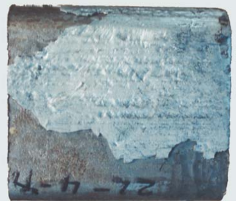
This small RHS section has severe galvanized coating delamination arising from very high phosphorous levels in the steel, creating a thick, fragile coating almost 1000 microns in thickness.
