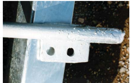
Weld splatter left on the steel will be galvanized along with the work, resulting in a rough and pimply appearance.
