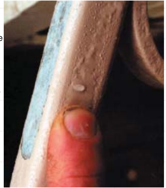
Poor surface preparation (no primer used) combined with paint application on damp galvanized steel resulted in this paint failure caused by water blisters under the paint film.
